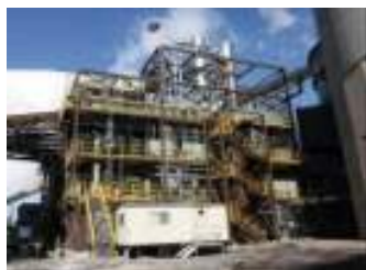
We Energies Pleasant Prairie USA - 5 MWth Chilled Ammonia - Coal
