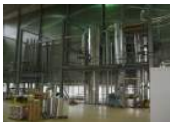
EoN Karlshamn Sweden - 5 MWth Chilled Ammonia - Fuel/Gas
