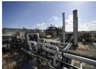
Total Lacq France - 30 MWth Oxy - Gas/Fuel
