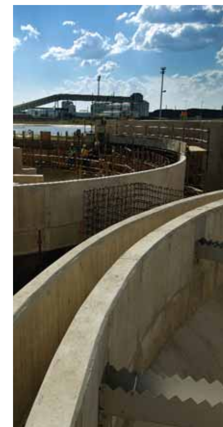
The Emalahleni Water Treatment Plant. Photo courtesy of Anglo Coal.
