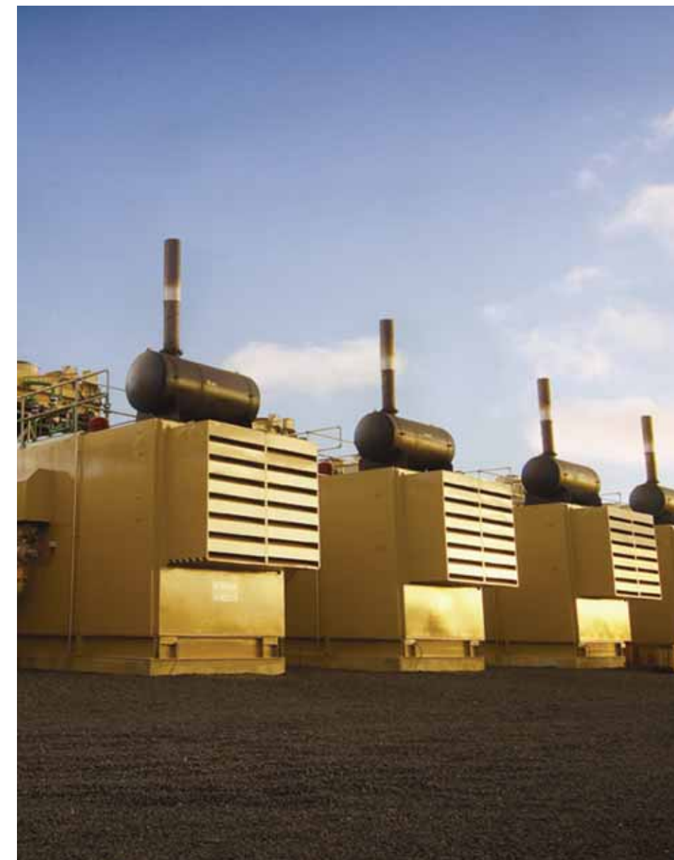
Oaky Creek Envirogen Plant, Photo courtesy of Xstrata Coal
